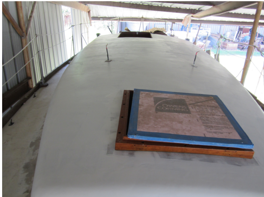
Cabin top after new fiberglass installed and in process of being sanded smooth for painting
